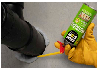
PVC Pipe Penetration
