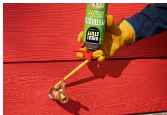
Water Faucet Penetration
